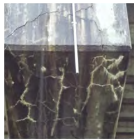
Discharged ASR gel through cracks: macroscopic motion
