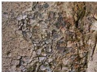
Disintegrated concrete after fatigue + stagnant water
