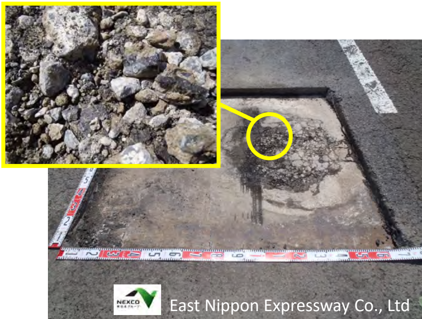
Aggregation on Highway bridge deck
