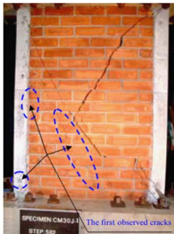
Final crack pattern (Experiment)
